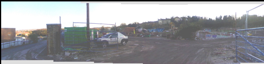
ABOVE: This photo shows the site of the Abattoir in the course of demolition on 21st November 2006. This is the view looking back towards Lewes Road. The junction of Mayo Road and Princes Road can be seen on the horizon in the background. The Abattoir building would have stood to the right of the bush, dead centre of the photo. The Pillar in front of the Landrover is part of the front wall of what was originally a weighbridge hut, seen in the centre of the photo in the link, HERE . (TBA)
