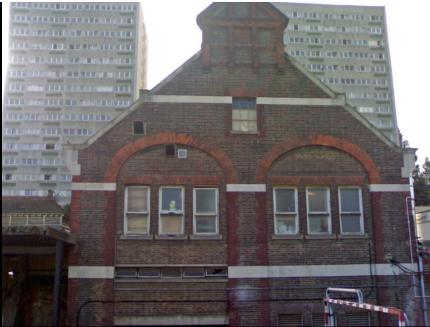
ABOVE: This shot of the front of the building shows how little the structure has changed since it was built: apart from the changes to the windows and the removal of the iron gantry adjoining the frontage, relatively little has changed in 60 years.
