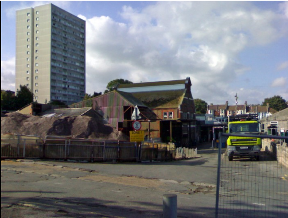
ABOVE: 3/4 view of the remaining Dust Destructor buildings looking roughly due north. The chimney would have been just to the right of the circular sign / zone 1 sign in the centre of the photo.
